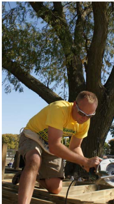
Aviva employee Joe Riesberg builds foundation for a backyard deck at Youth Emergency Service & Shelter.
